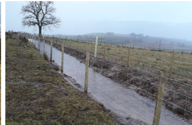
Figure 3. Recently constructed cross-slope swale prior to vegetation establishment, with downslope low level bund and fencing to protect from poaching © West Cumbria Rivers Trust
