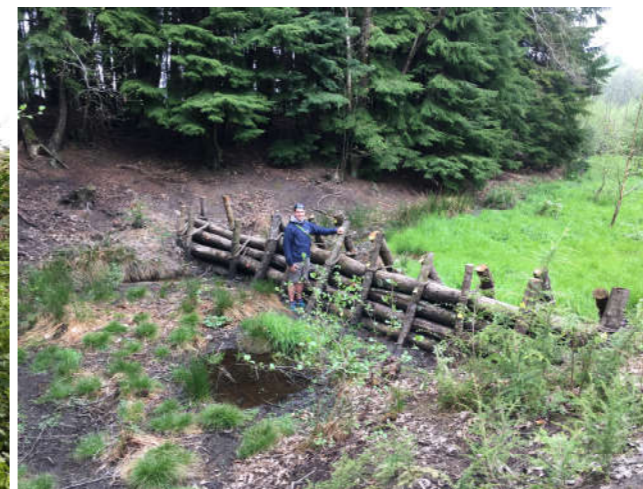
Figure 2. A multiple log overland leaky barrier, with extended in-channel leaky barrier (WC01.1) and substantial fixings (© Jay Neale)
