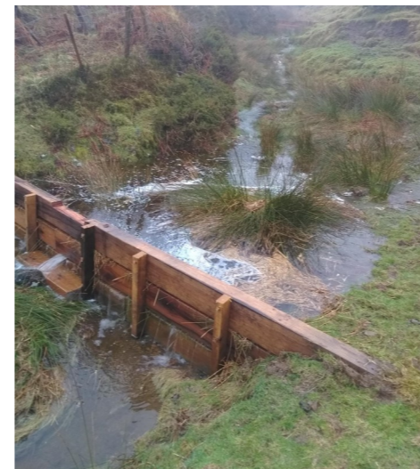
Figure 2. Formal leaky wooden dam blocking a moorland gully (© Dartmoor National Park Authority (DNPA), © Environment Agency)
