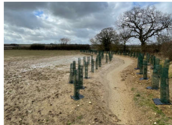
Figure 2. Recently constructed cross-slope swale at field edge with tree planting, as part of the Evenlode NFM scheme © Dave Gasca-Tucker
