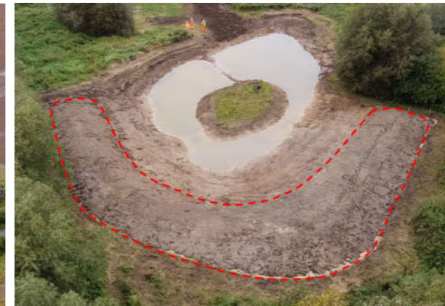
Figure 2. A newly constructed containment bund (with red dashed line) in conjunction with offline storage pond as part of the River Soar NFM Pilot Scheme (© Atkins Ltd)
