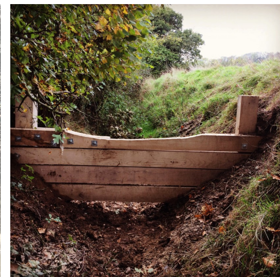
Figure 4. Formal in-channel leaky barrier constructed from wood planks, located above the base flow level and with notch in the top to allow spillage of high flows (© Shropshire Wildlife Trust, Kirsty Brown)
