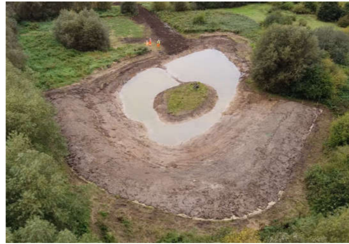
Figure 1. A newly constructed offline storage pond as part of the River Soar NFM pilot scheme (© Atkins Ltd)
